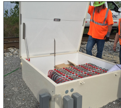
(20) SUN+660 Batteries & Battery Box
